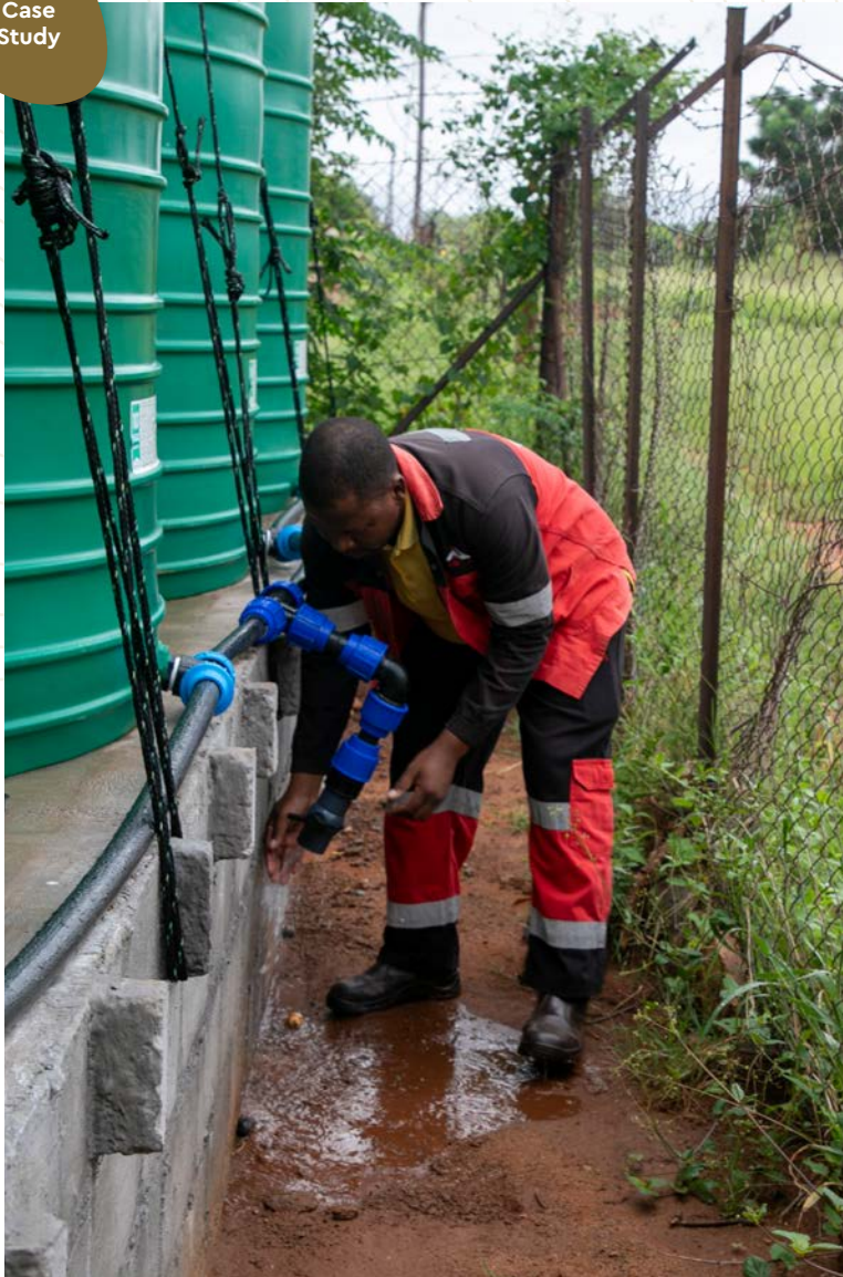
Water supply stations provide potable water for essential needs
