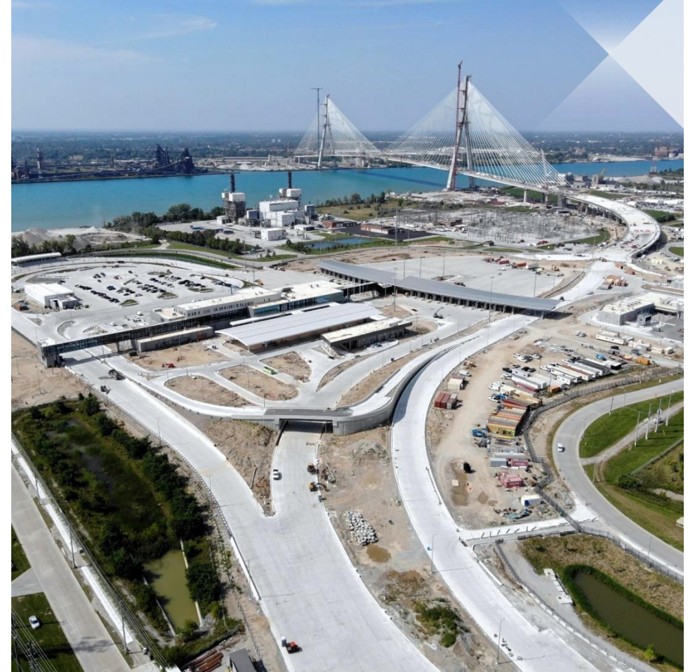
GORDIE HOWE INTERNATIONAL BRIDGE // PORTS OF ENTRY INTO CANADA AND THE U.S.
