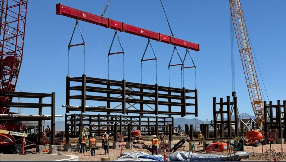
Pipe Rack Modules south of Cation Removal Ion Exchange Building
