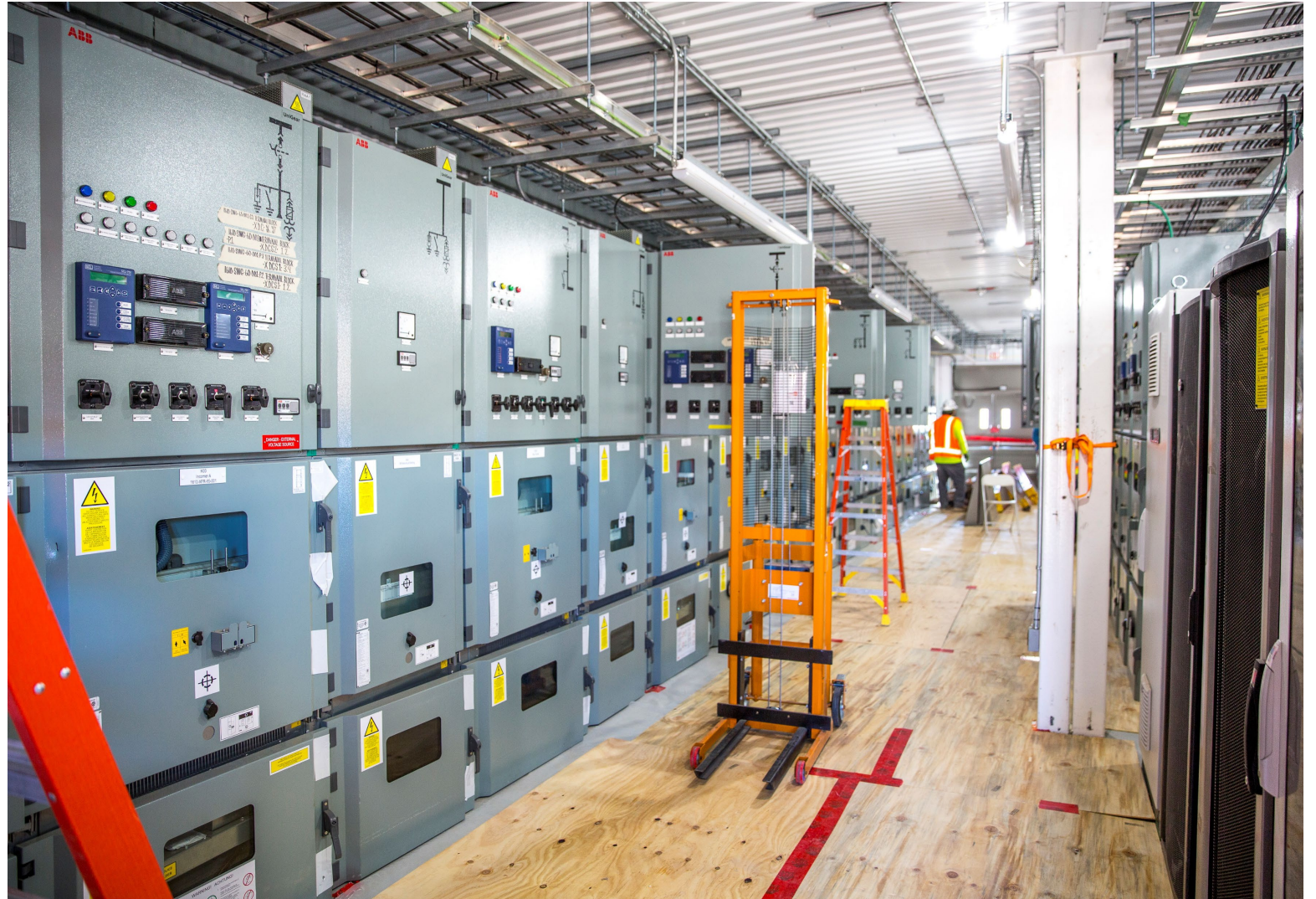
Inside one of the electrical houses (E-House), a prefabricated building housing electrical control systems
