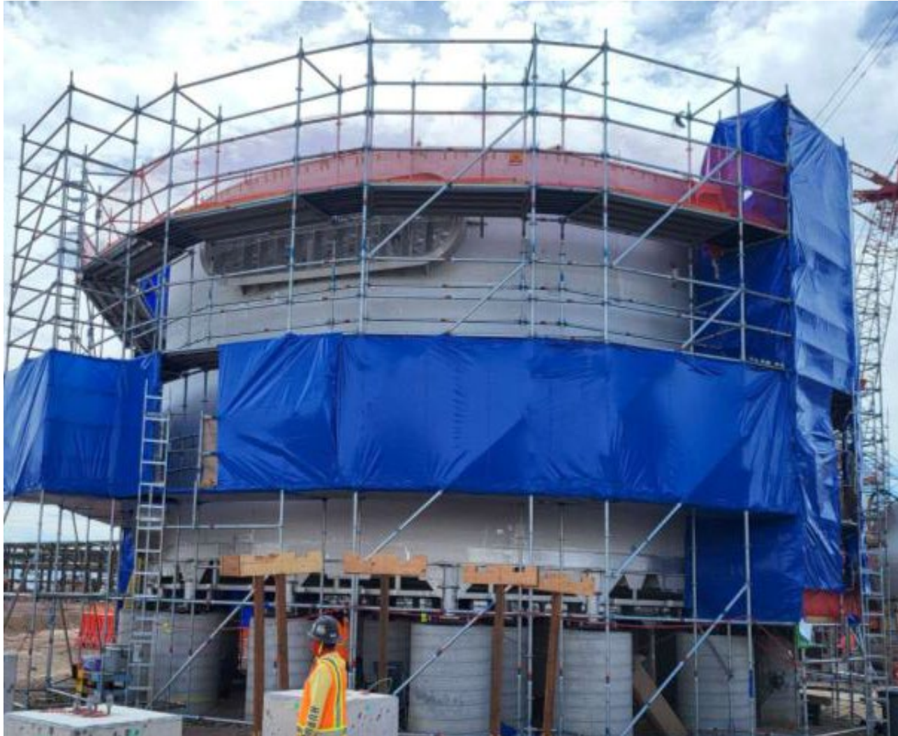
The Sulfuric Acid Plant's stainless-steel converter installation
