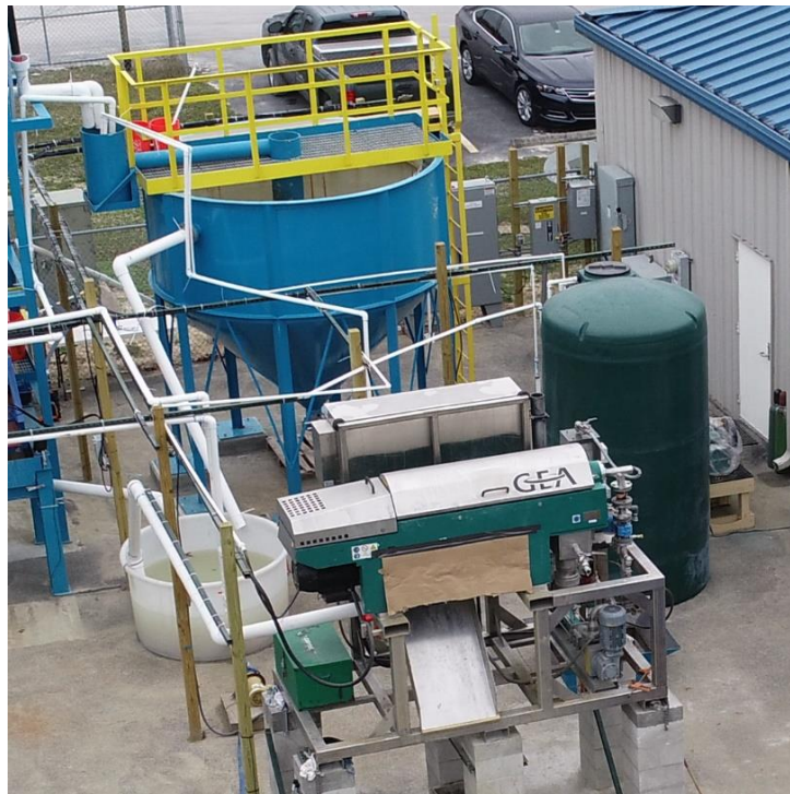
Figure 13-11 Thickener and Decanter Centrifuge
