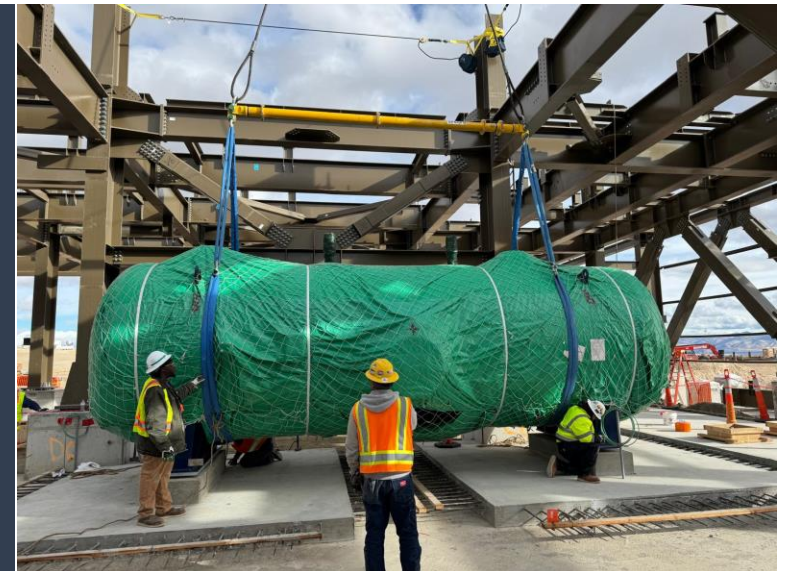
Air receivers were safely lowered into the Filter Building
