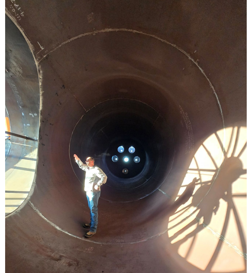
Inspecting the transition piece that will be installed once it arrives at Thacker Pass
