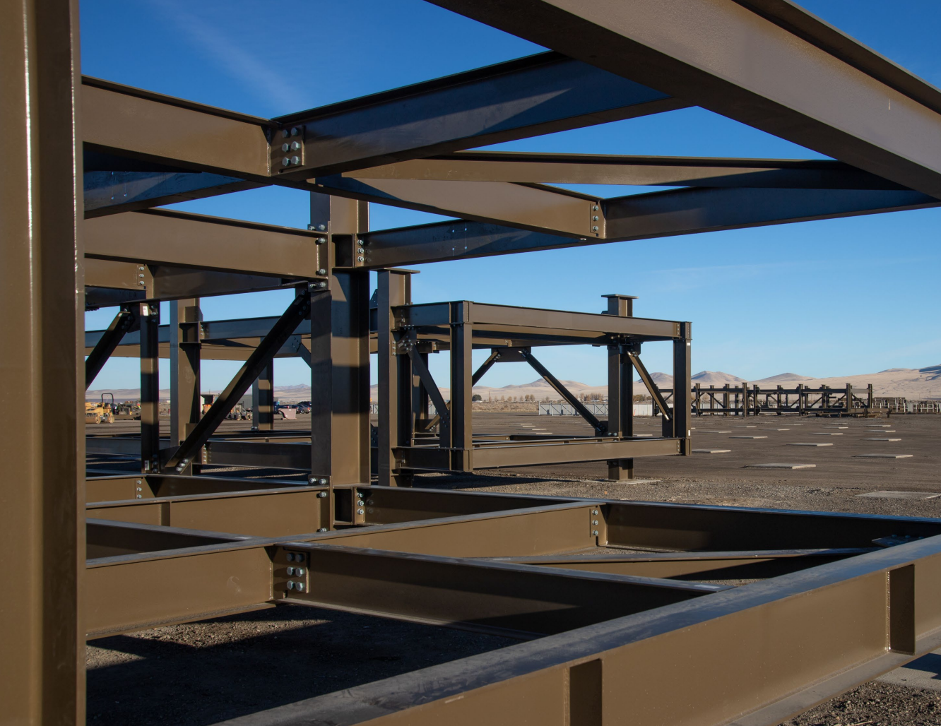
Over 90 pipe rack modules will be assembled in Winnemucca at CarWil for installation at site
