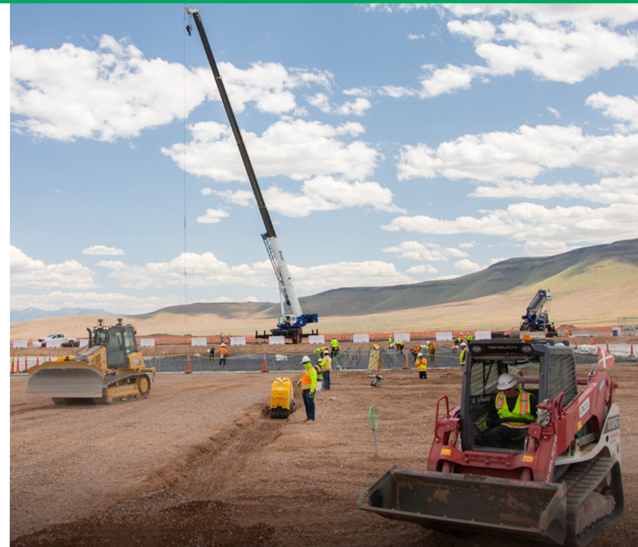
Preparing Thacker Pass for the buildout of Counter-Current Decantation (CCD) thickener tanks.
