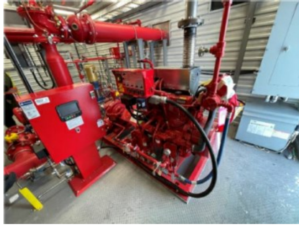
Figure 15-5 Fire Water Pumping Module
