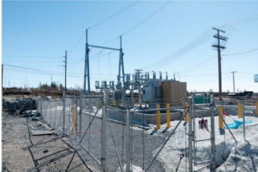
Figure 15-13 New Electrical Room and Transformer Bay
