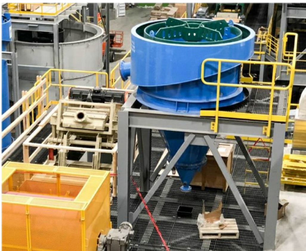
Figure 21-9 View of the Hydrocyclone
