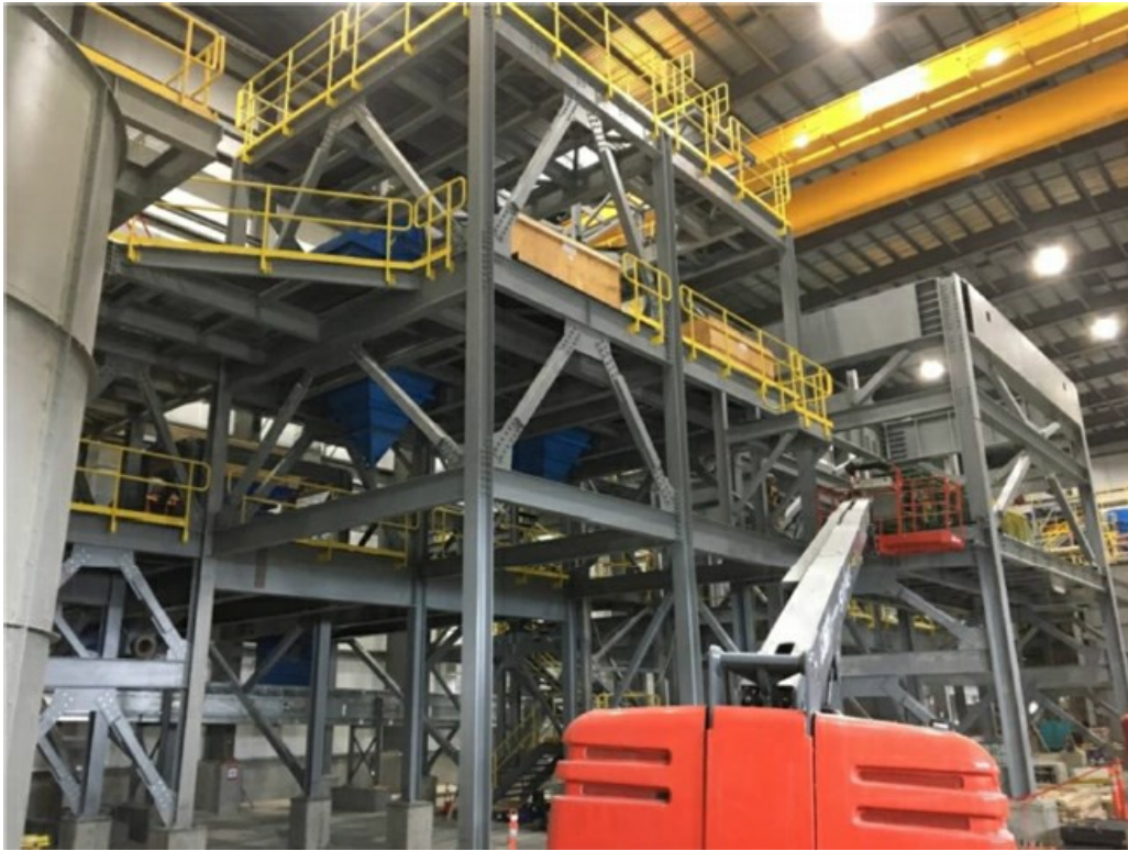
Figure 21-10 View of the Hydraulic Separators
