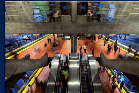
Heavy duty public escalators Montréal metro
