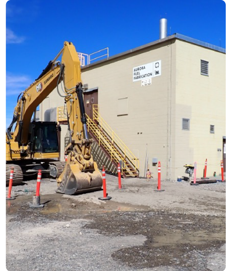
Oklo's Aurora Fuel Fabrication Facility (Images: Oklo)
