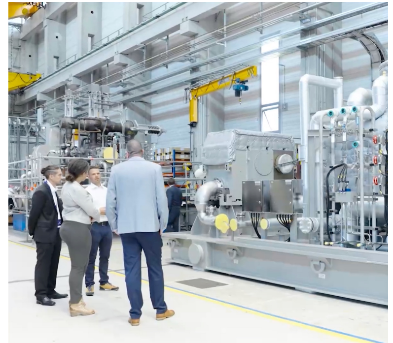
Alex Renner, Chief Product Officer, and Scott Auerbach, Director of Power Engineering, engage in a discussion of the industrial steam turbine package with the Siemens Energy team.
